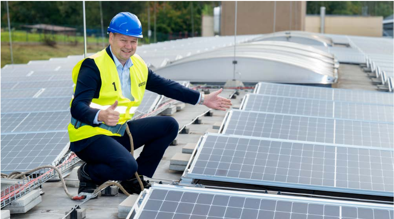
Pavel Kubicek, Head of Operations, Rieter CZ, presents the latest photovoltaic system at the Ústí nad Orlicí location in the Czech Republic.
